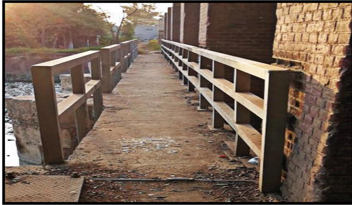
Plate No. 7: Viaduct with an iron balustrade adjacent to the front façade of the Bagouria barrage (Photographed by the researcher).
