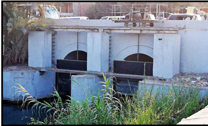
Plate 19: A general view showing the eastern front façade of the Sersawya barrage (photographed by the researcher)
