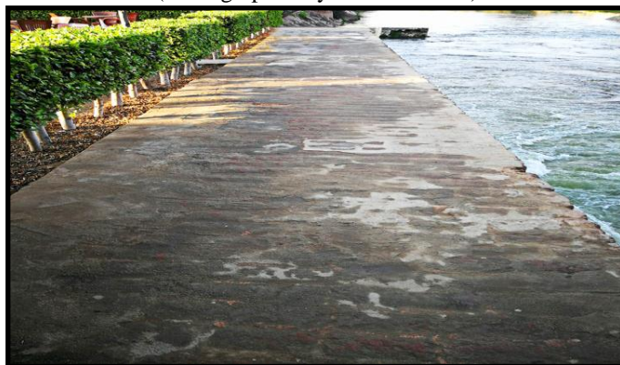
Plate No. 21: The western pavement of the weir of the Bagouria barrage. (Photographed by the researcher)
