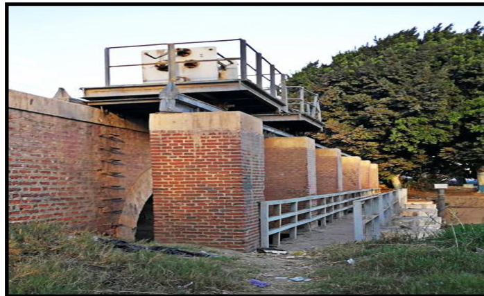
Plate No. 8: Viaduct and the shoulders located on the front façade of the Bagouria barrage (Photographed by the researcher).
