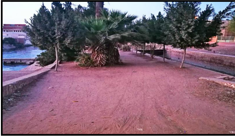
Plate No. 25: The embankment between the weir and the lock from the back side (Photographed by the researcher).
