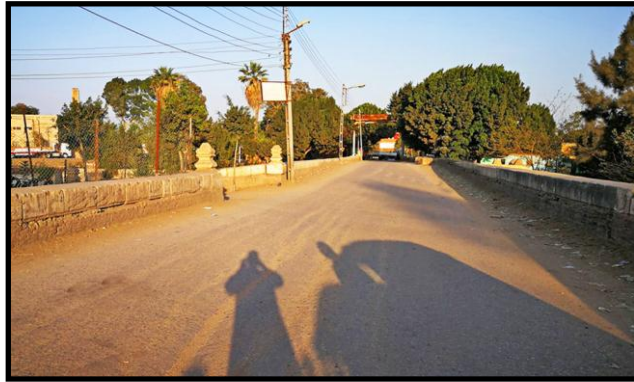
Plate No. 22: The upper road of the Bagouria barrage. (Photographed by the researcher)
