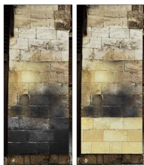
[FIGURES 15/A-B]: A. Shows the blackened wall before treatment; (B). The cleaned area after chemical–biological treatment © Photo taken by the researchers
