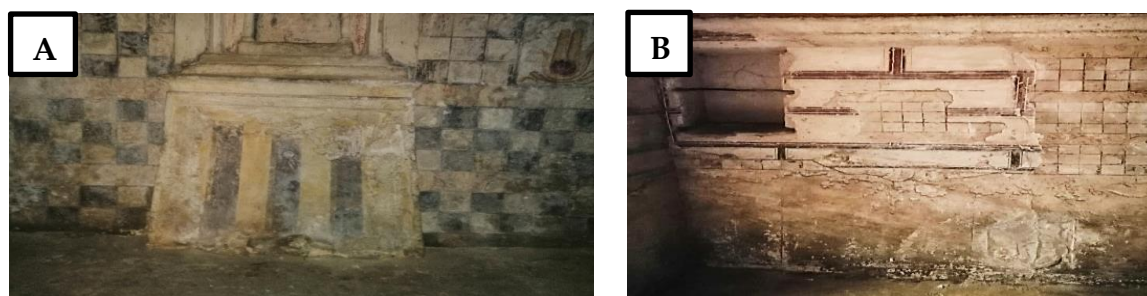
[FIGURES 3/A-B]: Areas for sample collection; A. Fading pigments and salt efflorescence on the surface; B. Broken film layers with a growing fungus in the regions near the ground © Photos taken by MOHAMED ABD ELRAHIM
