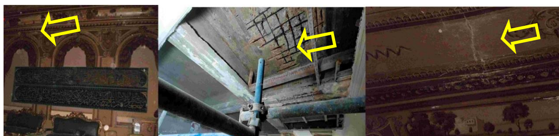
[FIGURE 6]: Structural deterioration in the walls and ceiling of the Kiswa Hall , showing the location and extent of cracks marked by the arrows © Photos taken by TAHA ATALLAH
